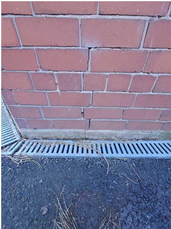
Image 1: Cracking in exterior wall
